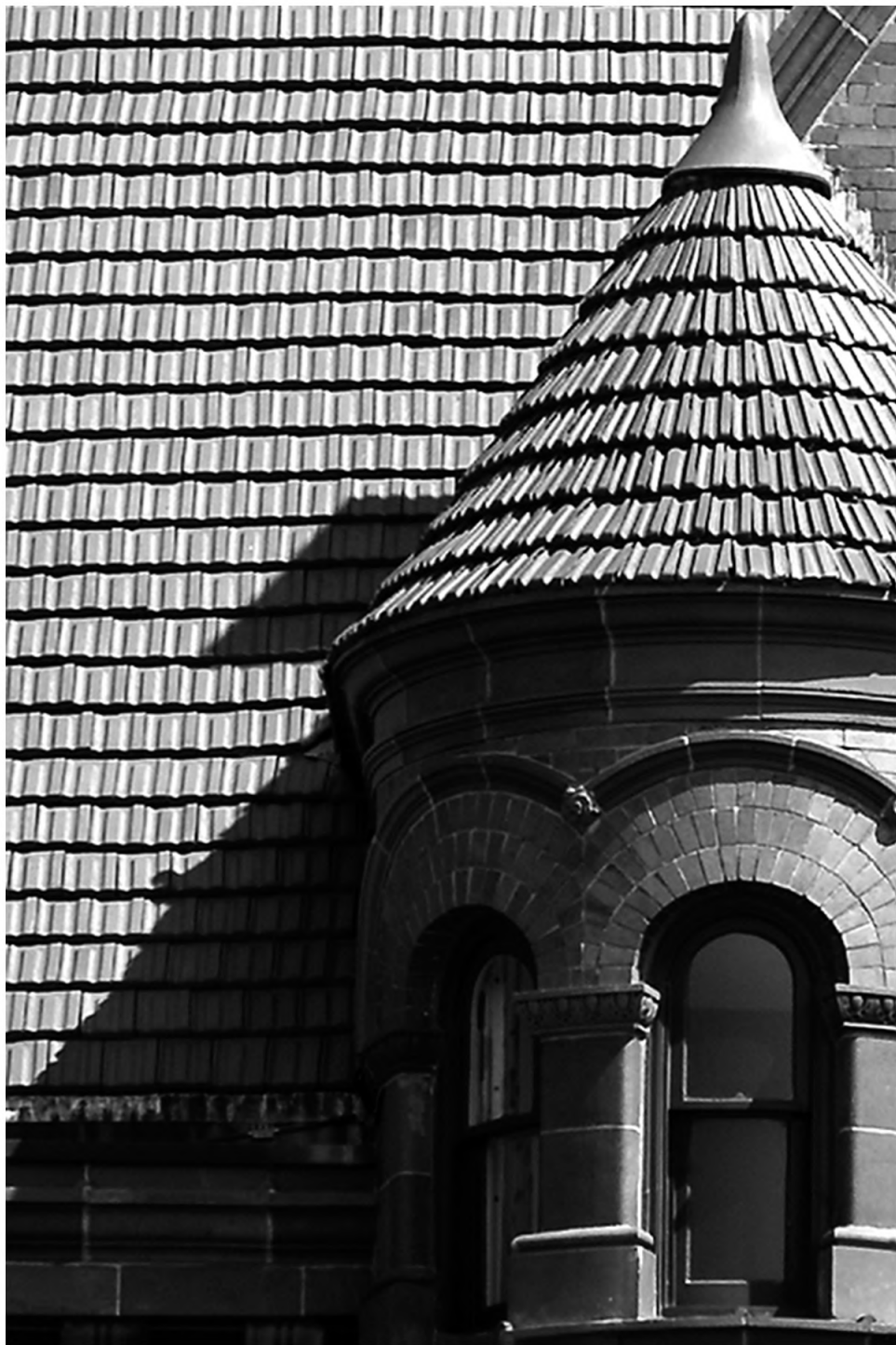
Former DuPage County Courthouse, Wheaton, IL, Roof Details, 2021 Pigment Print Print size: 8 x 12 inches Frame size: 12 x 16 inches
