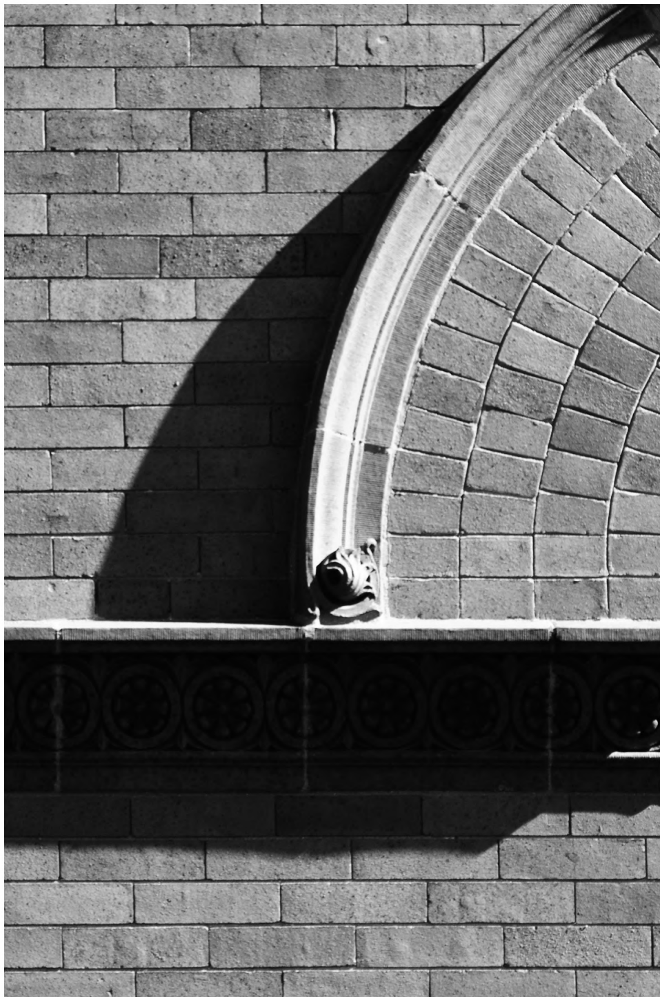
Former DuPage County Courthouse, Wheaton, IL, Architectural Detail, 2011 Pigment Print Print size: 8 x 12 inches Frame size: 12 x 16 inches
