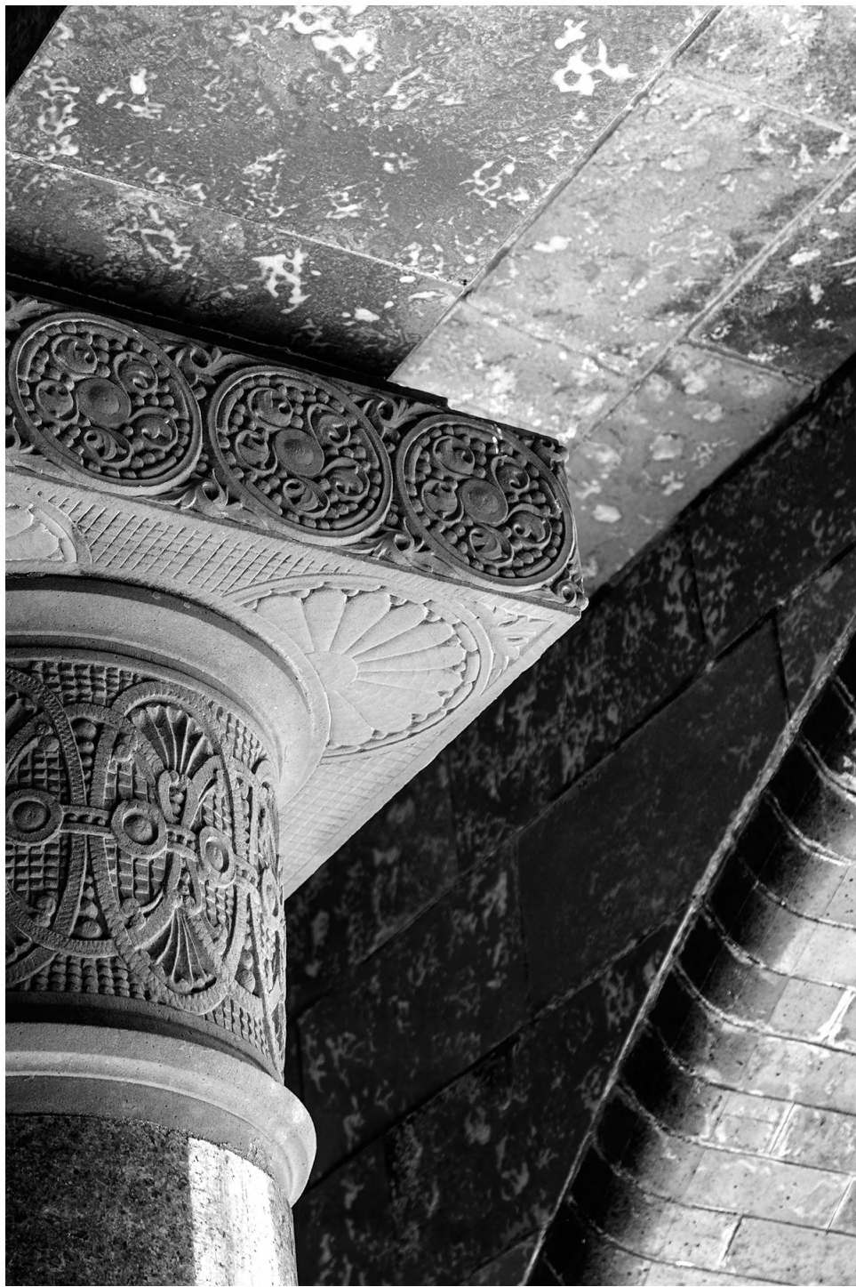
Former DuPage County Courthouse, Wheaton, IL, Column Details, 2017 Pigment Print Print size: 8 x 12 inches Frame size: 12 x 16 inches
